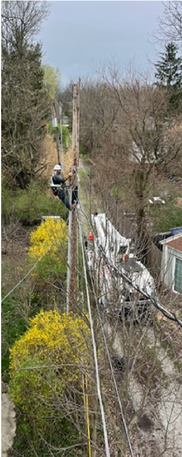
Recent electric department projects.
